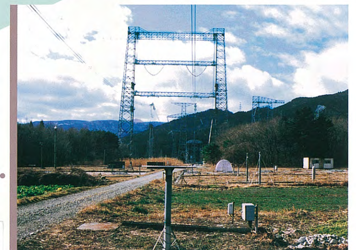
Test line and ion flow measurement devices
