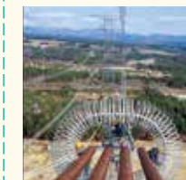
UHV AC test transmission lines
