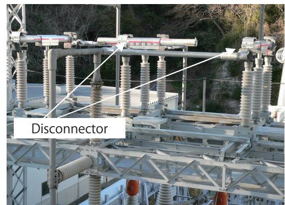
Photo 2: 115kV Horizontal Break disconnector (3-unit interlock operation)
