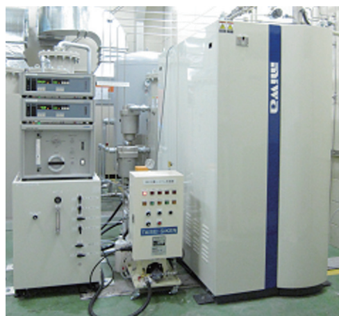
Photo 2: Appearance of low-concentration CO 2 -generating equipment
