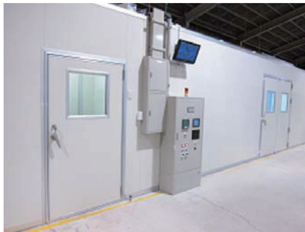
Photo 1: Appearance of an airtight constant temperature and humidity room, along with the control and monitoring apparatus
