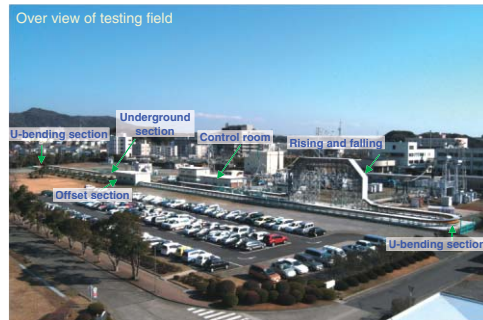
500-m HTS power cable testing facilities
