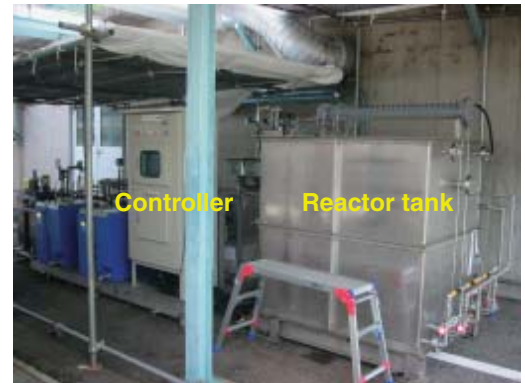
Photo.1 Large-scale system installed in thermal power plant
