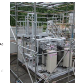
Fig. 2 Small-scale verification test using an actual-size superheating pipe (Kyushu/Takigami geothermal power plant)
