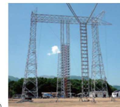
12 MV impulse generator (Shiobara Testing Yard)
