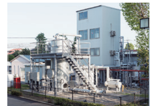
Test facility for Filtered Containment Venting System (FCVS) performance evaluation A full-scale test section and equipment such as steam boilers are also installed.
