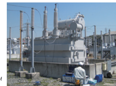
Diagnosis of abnormalities of transformer winding by FRA
